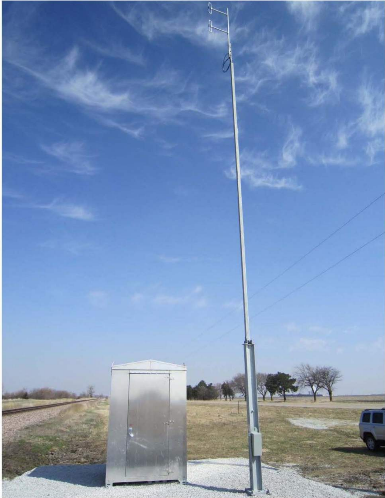
Figure 48. Photograph of a typical PTC pole installation with associated infrastructure.
